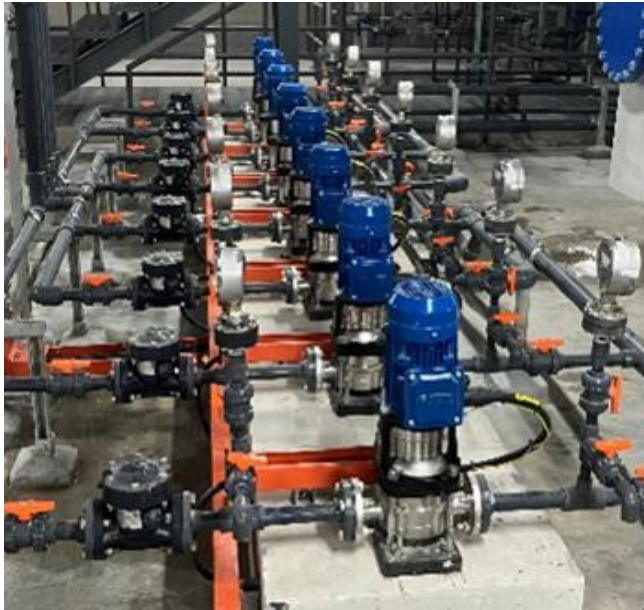
Booster System in Bidadari
