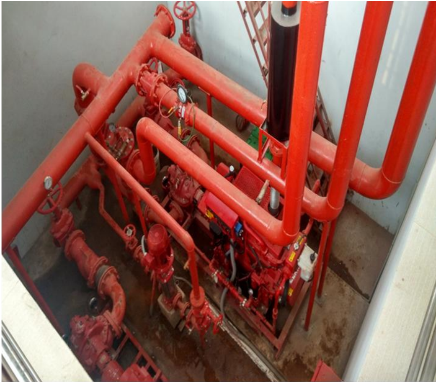
Completed Fire Fighting System in Bangladesh
